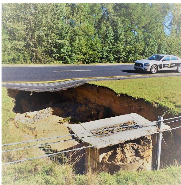
FIGURE 5.16: SINKHOLE IN NORTH CAROLINA
